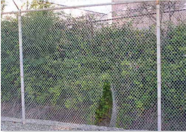
A typical perimeter security breach. Photo courtesy of BC Hydro.
